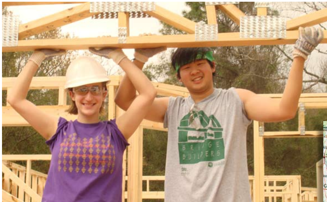
Urania Dagalakis 09OX and Kevin Szu-Tu 09OX work on framing as part of the Habitat for Humanity project in Mobile, Alabama.
